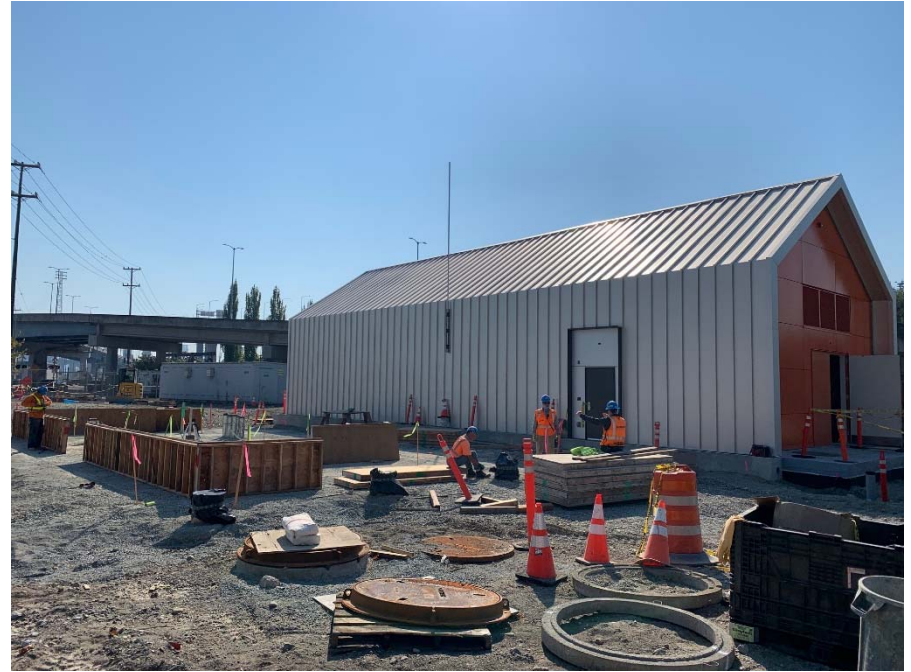
Seattle City Light Pads at Substation
